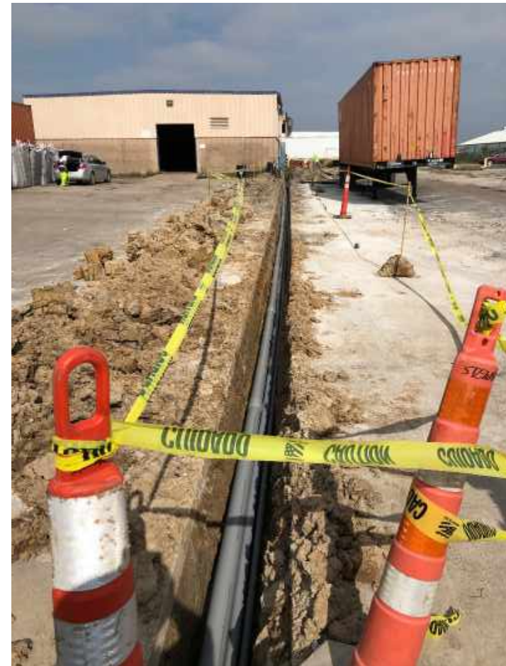
Underground conduits at parking lot.
